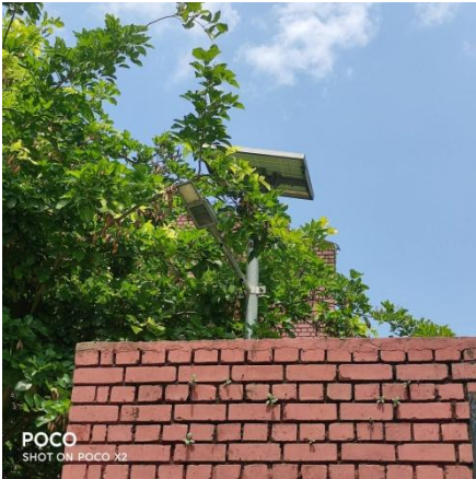
Figure 3 Use of Solar Energy
