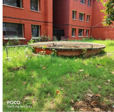
Figure 2 Rainwater harvesting tank
